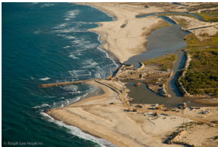
Construction that has already begun on nearby Cabo Riviera shows heavy equipment and dredges working in the estuary at the mouth of the San Dionisio wash, the town of La Ribera's freshwater source. This is one of the windiest sections of the Baja coast and erosion is already taking its toll. photo: Ralph Lee Hopkins/LightHawk
