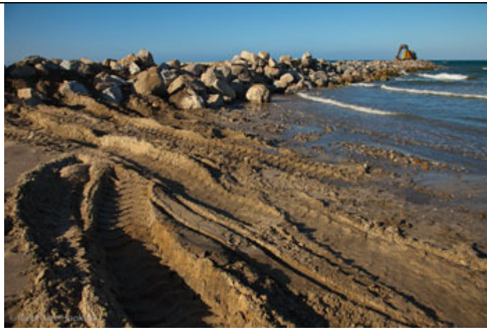
Evidence of heavy machinery on the ground at the Cabo Riviera development site. photo: Ralph Lee Hopkins/LightHawk
